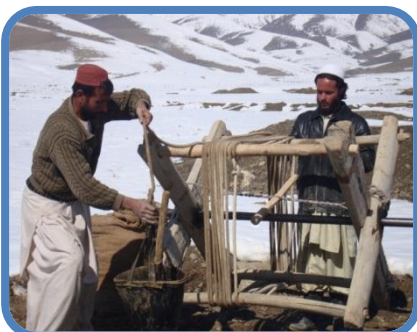
Cleaning the Qala-e-Sorkh Karez in Sayed Abad. Operator uses winch to haul buckets of debris from the karez and lower tools to workers
