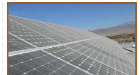
Thirty solar panels deliver a continuous power supply to the district's main office. Meanwhile, solar irrigation pumps deliver water to planted areas and buildings from an on-site reservoir at virtually no maintenance cost.
